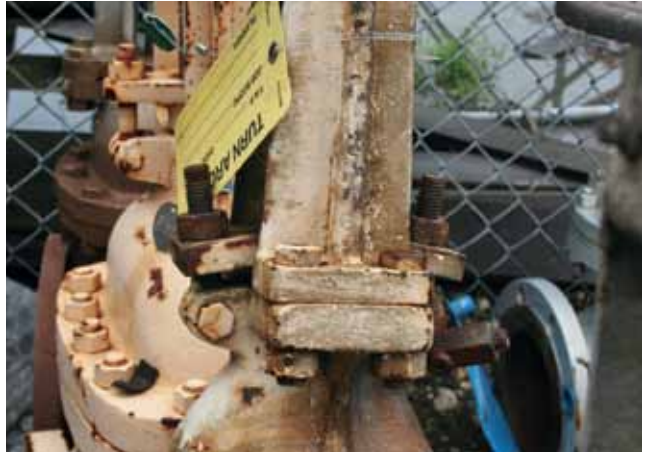
Image 1. Example of unacceptable packing gland conditions
