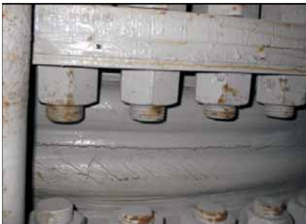
Figure 1. Typical Expansion Joint Surface Cracking
