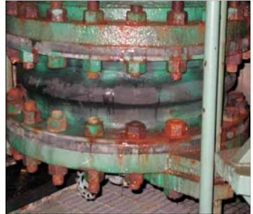
Figure 3. Leaking Expansion Joint
