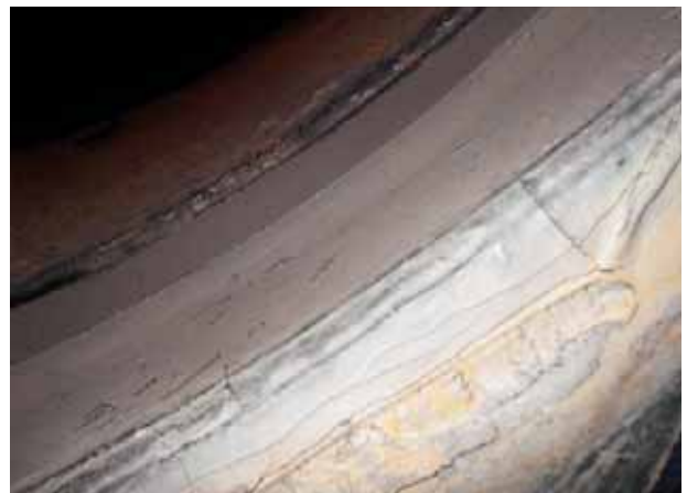
Figure 2. Expansion Joint Surface Delamination
