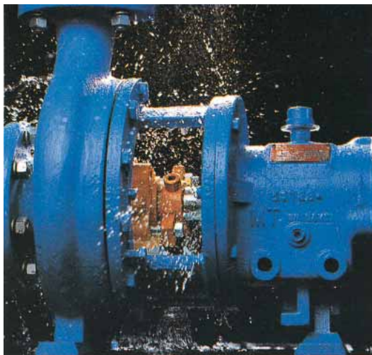
Figure 1. A typical pump packing failure.
