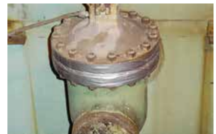
IMAGE 2: Flanged gasket with duct tape to identify air ingestion
