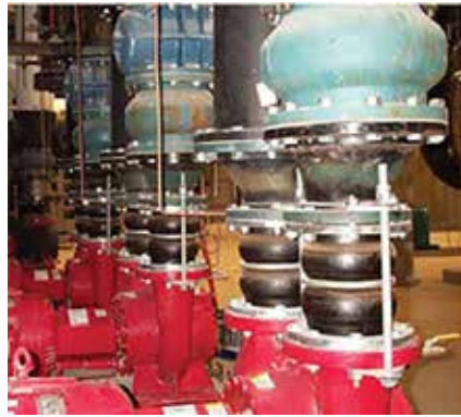
IMAGE 7: Typical rubber joint pump installation
